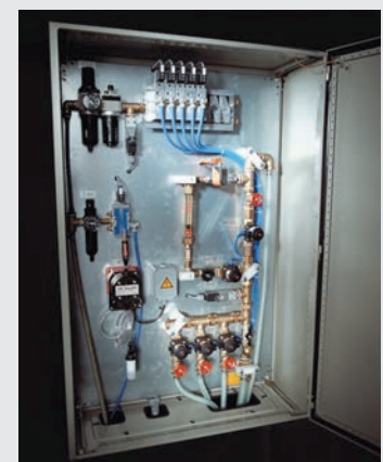
Compressed air distribution, process water and compound dosage
