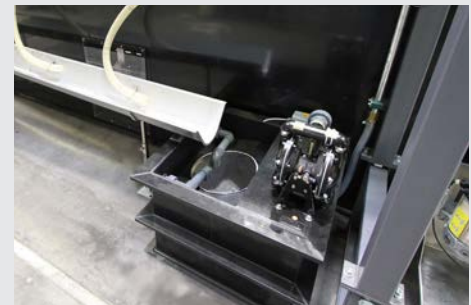
Process water collection chute with lifting station
